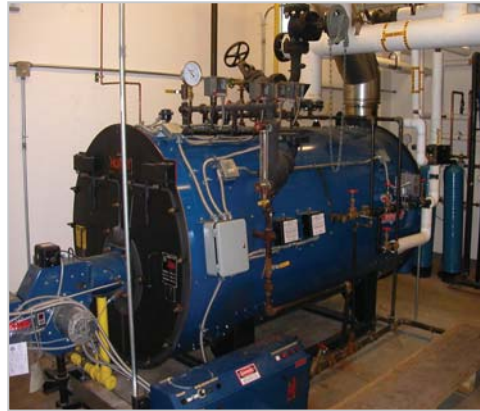
Medium Pressure Steam Boiler Plant
