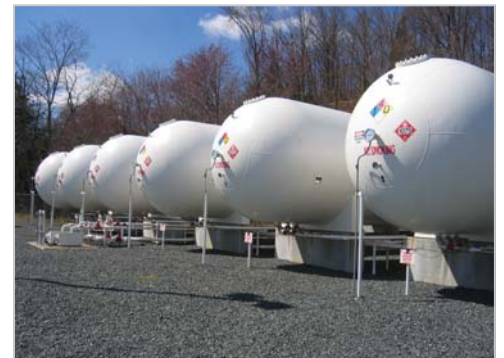
A propane/air system is used during curtailments. The propane system also enhances energy security as a back-up to the natural gas lines outside the fence in the event they experience a catastrophe failure.
